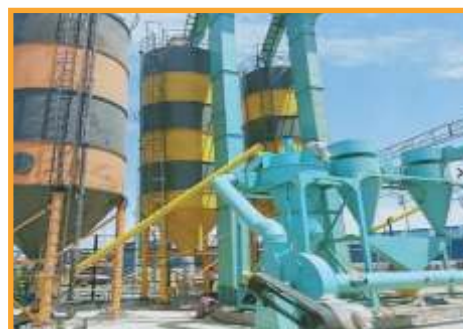
Fig 12: RMC Plant of UltraTech Cement Ltd.
