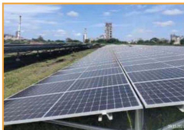
Fig 6: Solar Power Plant at J K Cement Ltd.
