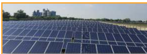
Fig 4a: Solar Plant at Nuvoco Vistas Corporation Limited
