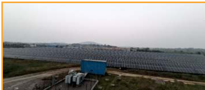
Fig 4: Solar Power Plant at Shree Cement
